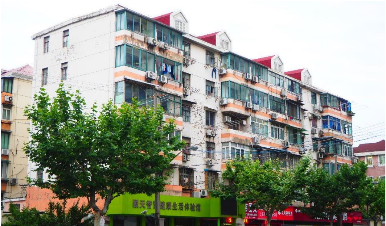
Figure 3-4 (below): Degraded façade of residential buildings.
