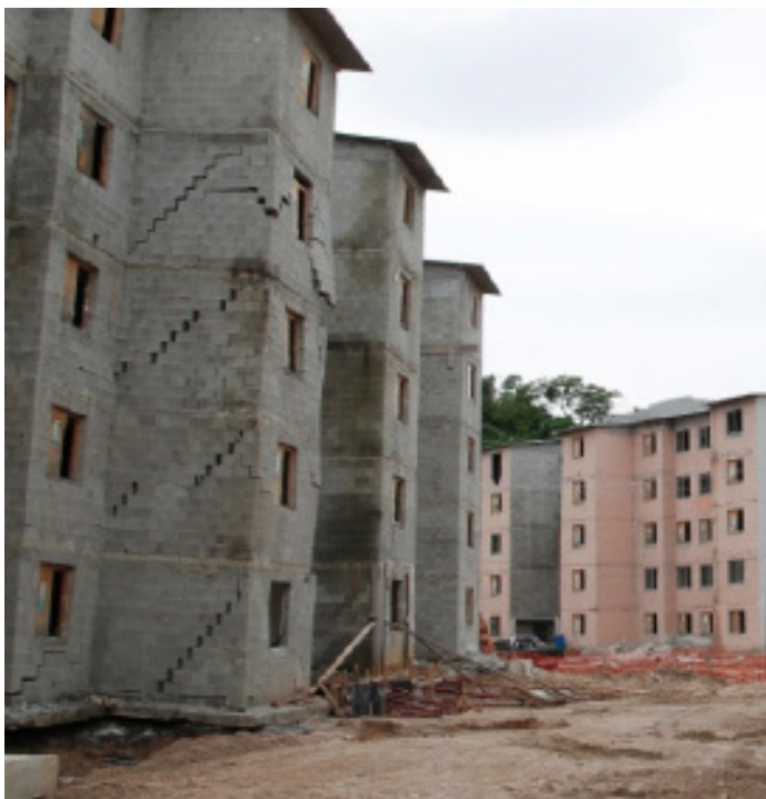
Figure 9. Crumbling MCMV housing in Niteroi, Rio de Janeiro Source: http://www.rioonwatch.org/?p=8023
