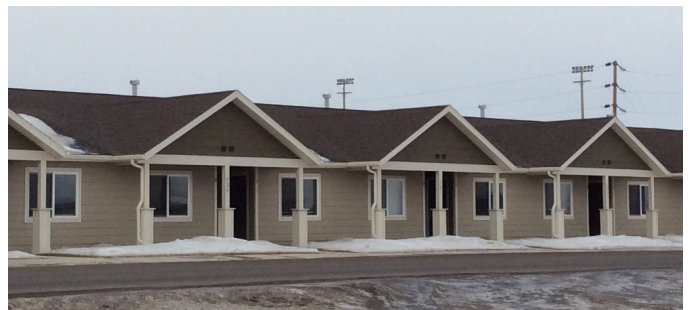
Photo: Permanent housing construction being built in January 2014 (time of site visit).
