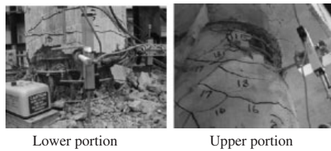
Figure 5. Damage observed on the lower and upper portions of Bent-3 after T-19.
