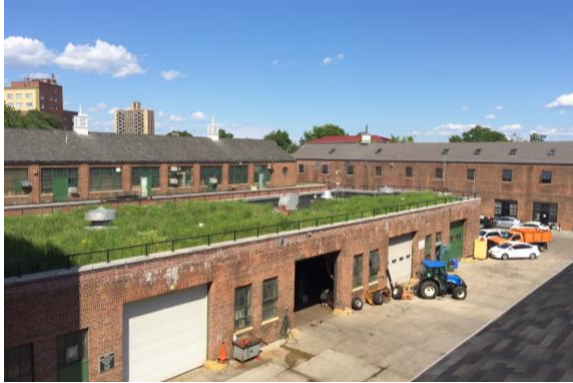
Figure 4.1 Ranaqua green roof is located above a NYC Parks auto garage in Bronx, NYC
