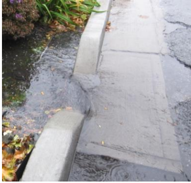
Figure 2.11 Efficient inlet design with concrete apron located in the street to slow down and direct water into ROWB 9B
