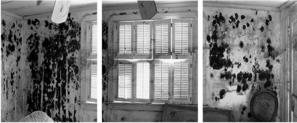
17. 6068 Louisville St. (mold), Lakeview, New Orleans, November 2006
