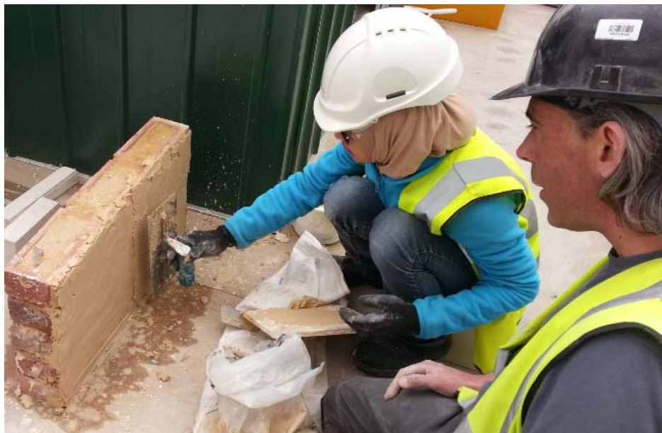
Figure 1-1. The author conducted a mini experiment under the guidance of the senior mason on site.
